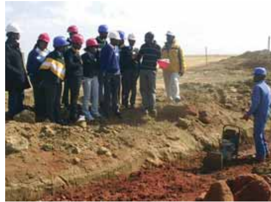
The contractor on site explains the preparation being done for the installation of bulk services.
